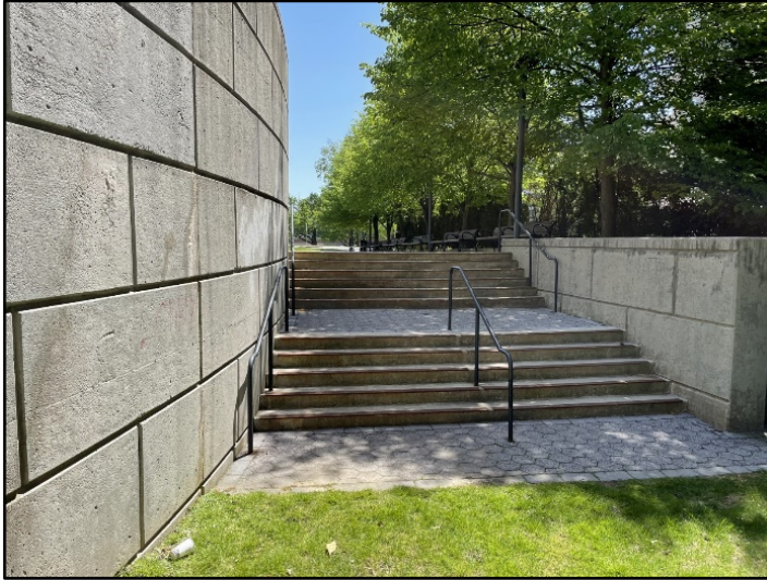
Missing Central Railing
