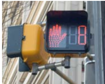
More countdown pedestrian timers were installed around the Village in 2007.
